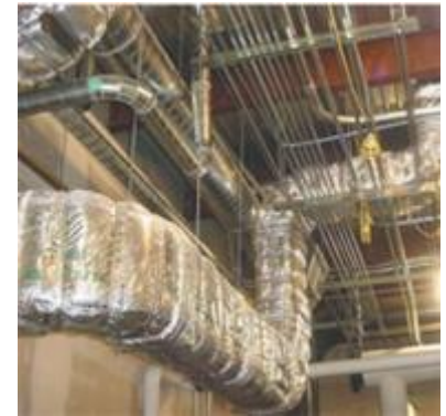
Internal Ducting in Cleveland Clinic Abu Dhabi
